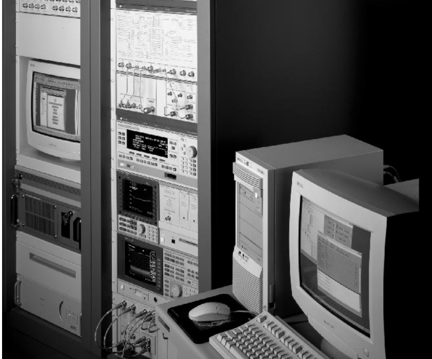
Agilent acceSS7 system used by Illuminet for network management.
